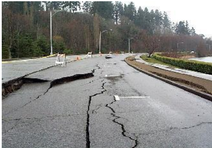
Figure 35 - Road damage caused by lateral spreading in Thurston County, Washington, an impact of the 2001 Nisqually Intraplate Earthquake. Photo – DOGAMI Archive
