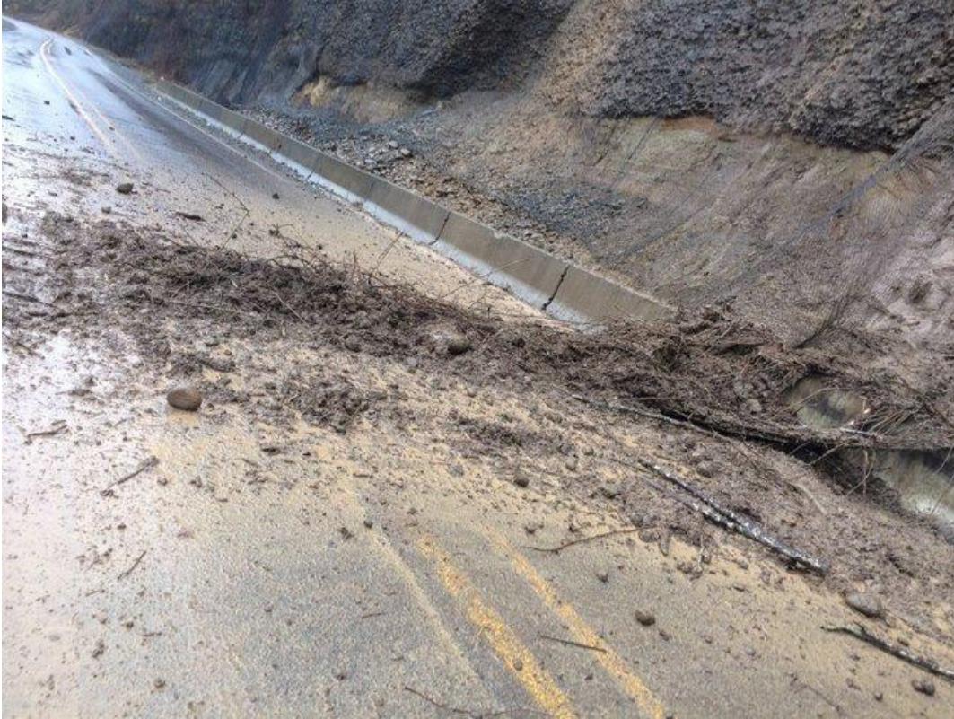
Figure 65 - Minor 2017 winter landslide on the East Historic Columbia River Highway. Photo Multnomah County Sheriff's Office
