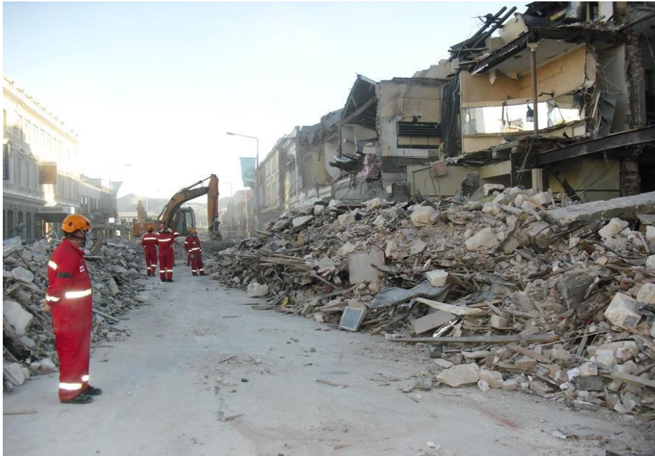
Figure 39 - Cleanup after the 2011 Christchurch Earthquake
