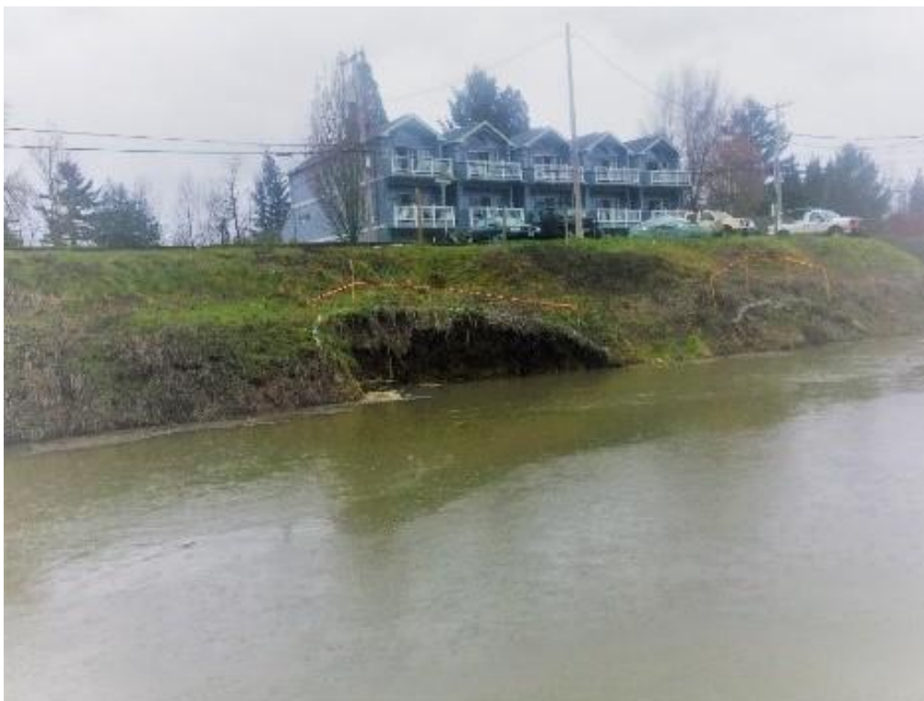
Figure 46 - Levee sloughing damage near NE Bridgeton Rd., in Portland caused by high water during the Spring 2017 flood event. Photo Multnomah County Drainage District.
