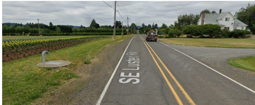
Figure 14. Example of Existing Air Vent and Access Vault (left) within Lusted Road ROW
