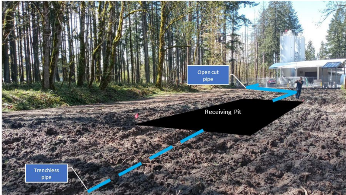
Figure 13. LRDM Receiving Pit in Lusted Hill Project Work Area (looking west), including Existing Cleared Utility Corridor Area in Foreground
