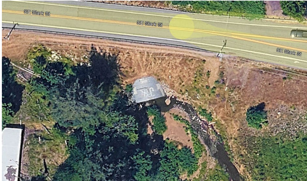
Figure 4-1. Upstream Channel Instability at Stark Street and Troutdale Road in Troutdale.
