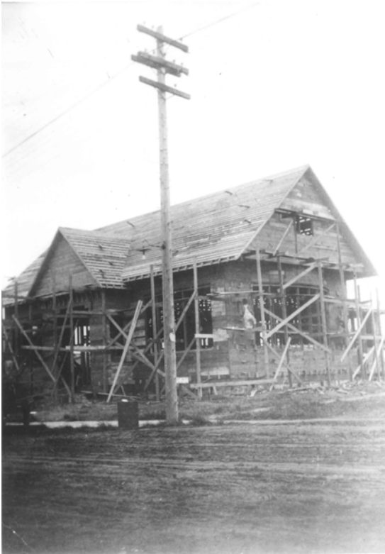
Copy of private print showing construction of original Gresham Branch Carnegie Library [1913]. From Department of Library Services accession 2002-000362/003, Branch Records.
