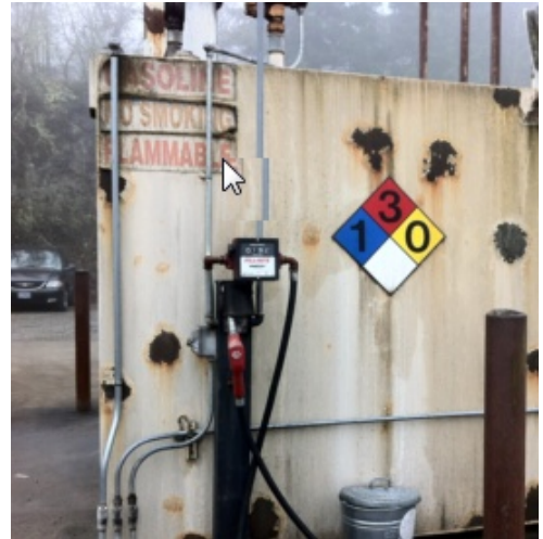
Bulk fuel pump at Skyline Road Shop Source: Auditor's Office
