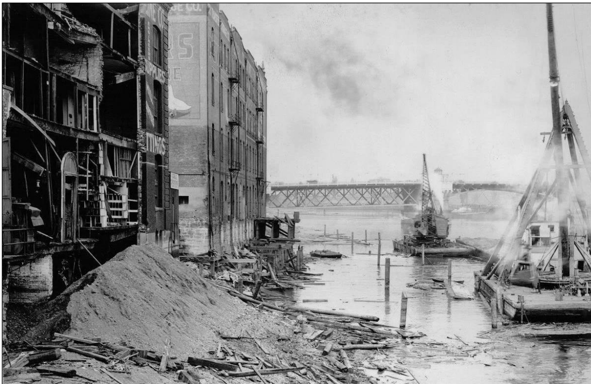
Figure 5-35. Preparation for Harbor Wall construction above the Burnside Bridge. Photo dated August 21, 1928.
