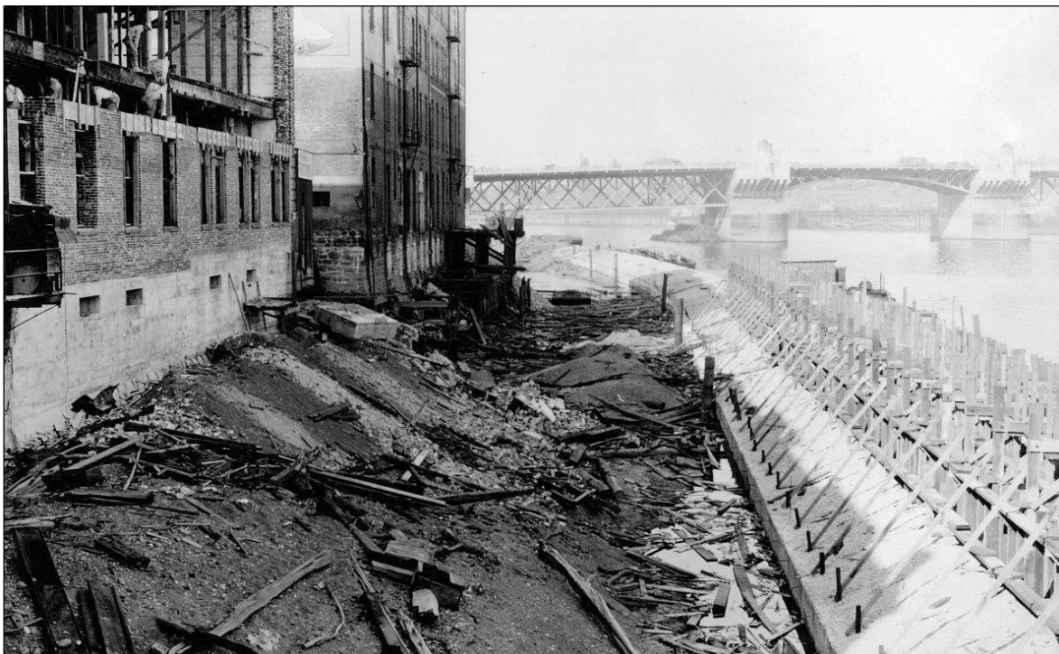
Figure 5-37. Construction in progress of Harbor Wall forms with view of debris on shoreline and reconstruction of rear wall of building damaged during dock removal on September 28, 1928.
