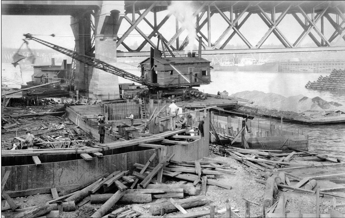
Figure 5-38. Construction of the foundations of the Ankeny Pumping Station. Current Burnside Bridge in background. Photo taken September 18, 1928.
