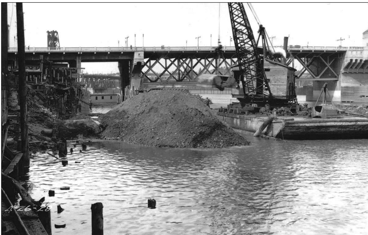
Figure 5-33. Stockpiling of dredged Harbor Wall fill immediately above the Burnside Bridge. Photo dated April 26, 1928.
