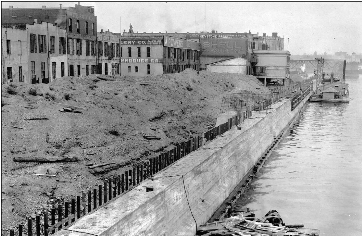
Figure 5-39. Construction of the Harbor Wall and surcharging of fill. Burnside Bridge is in the distance. Photo taken on October 16, 1928.
