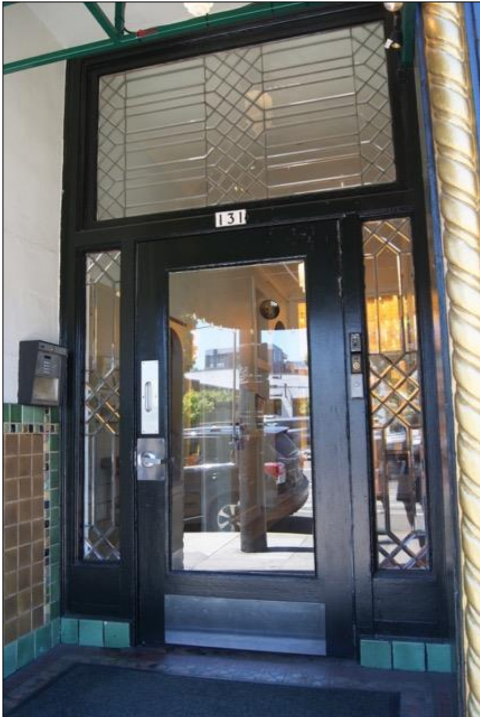
View: A detail of the main entry on the east façade showing the cable surround, colorful tile, and leaded glass sidelights and transom. The view is towards the west.
