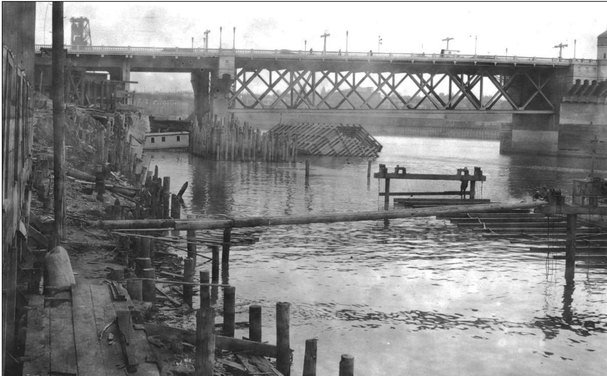
Figure 5-32. Dock remnants with continuing demolition in preparation of construction of the Harbor Wall, with the Burnside Bridge to the north. Photo dated March 8, 1928.
