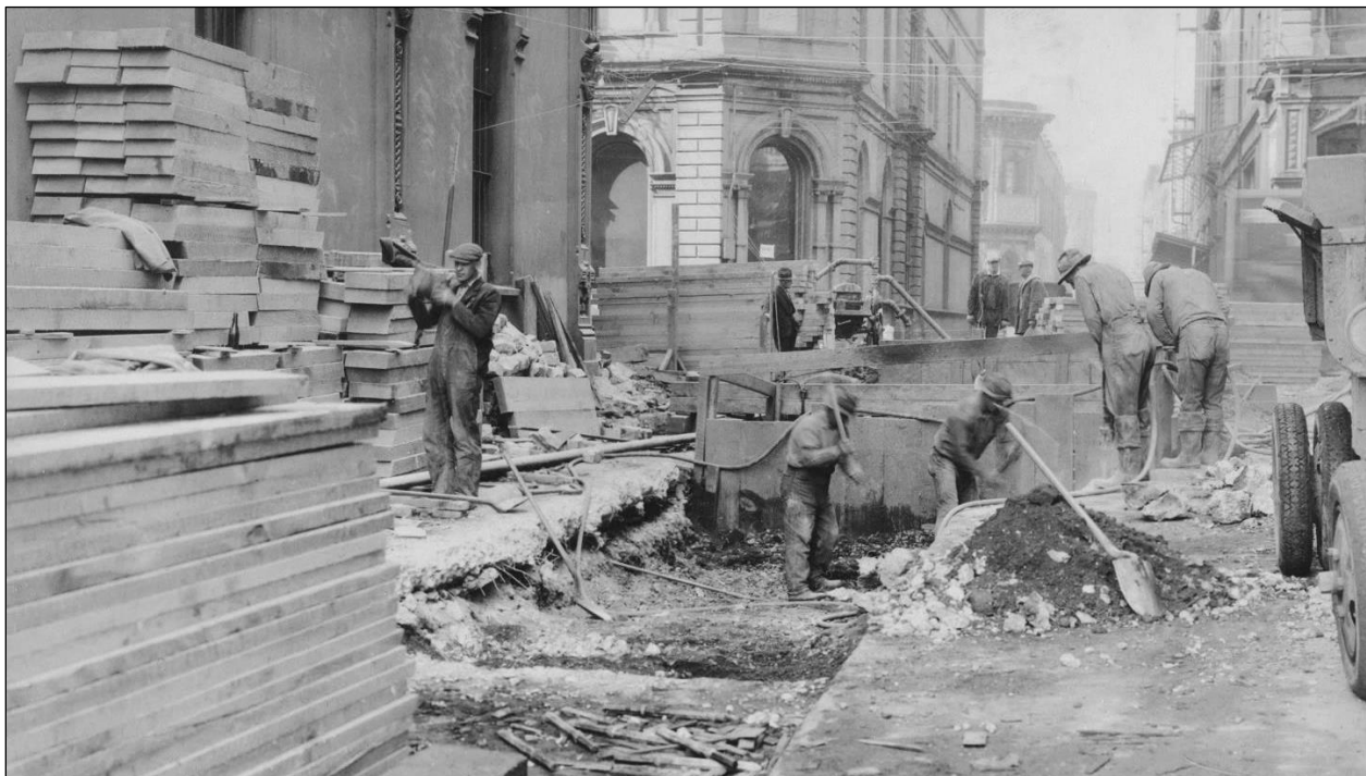
Figure 5-25. Open trench construction of the Front Street intercepting sewer, looking west along Ankeny Street to the intersection with Front Street. The trench is for the line extending to the Ankeny Pump Station. Photo dated 1928.
