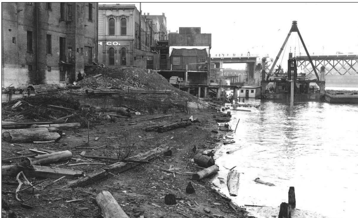
Figure 5-31. Clearance of docks and wharves in preparation of construction of the Harbor Wall, with the Burnside Bridge to the north. Photo dated January 31, 1928.
