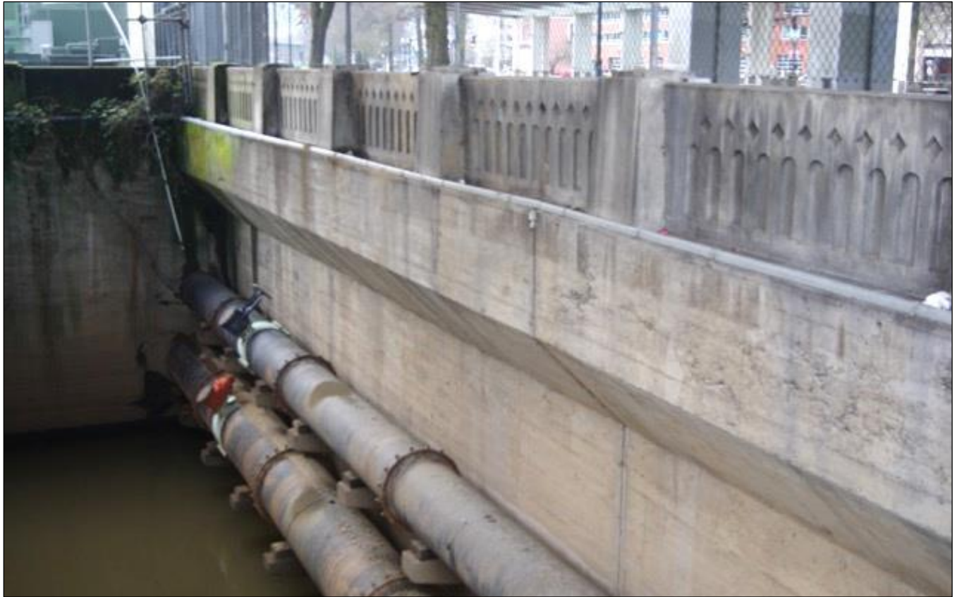
View: The Harbor Wall's original concrete bulkhead and railing where it faces Pier 1, view towards southwest.
