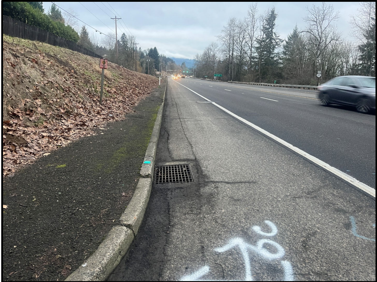
Slope on Northeast Edge of site adjacent to NW St Helens Rd, Facing Northwest
