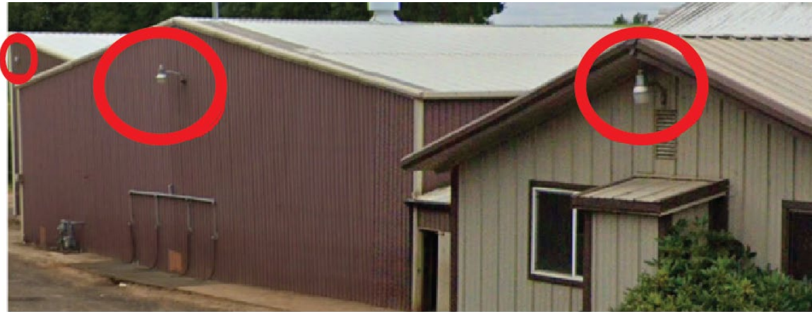
Figure 8. Unshielded Wall Lighting at Surface Nursery (Lusted Road)
