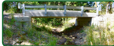
Top: Culvert blocks salmon trying to get home. Bottom: Bridge allows salmon to swim through.
