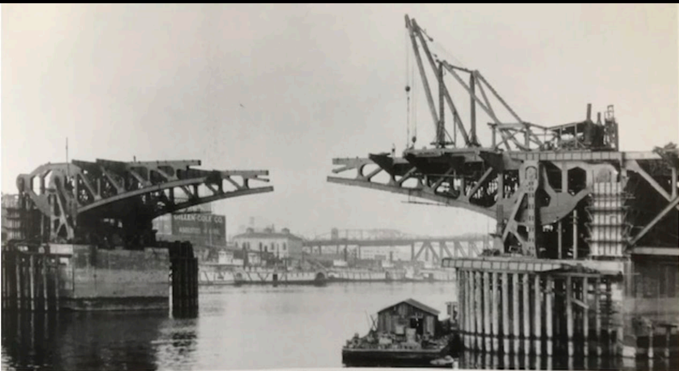
Portland Bridge bascule span construction, ca. 1925. Pier walls were built after the bascule leaves and counterweights.
