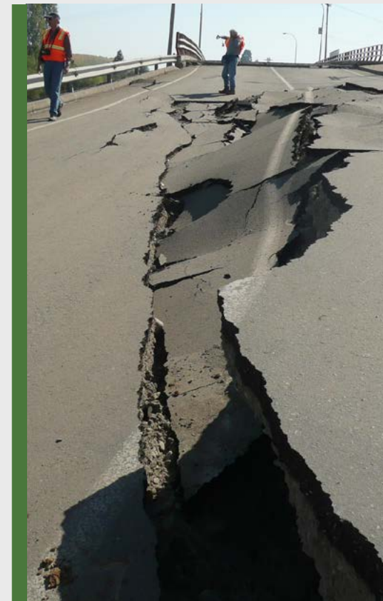
Damaged overpass approach
