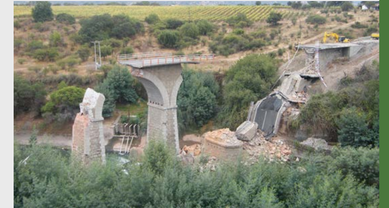
Collapsed bridge near Camarico
