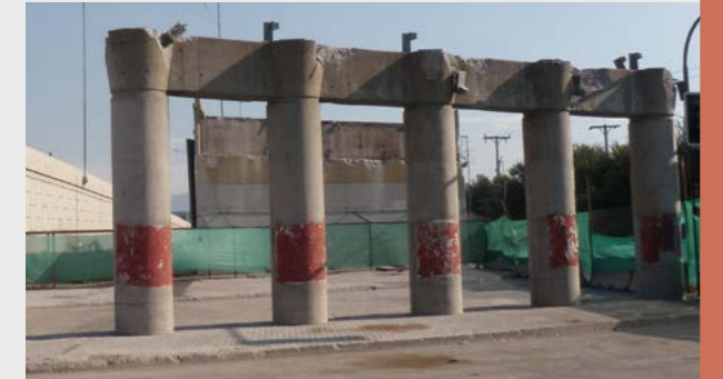
Remnants of collapsed bridge
