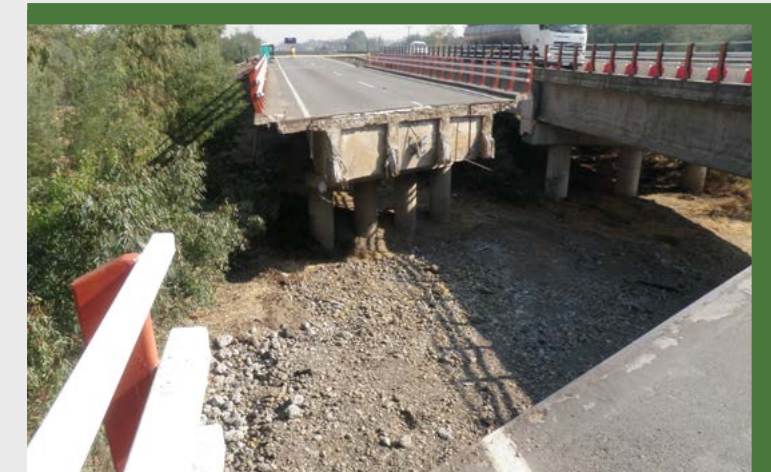
Damaged bridge south of Talca
