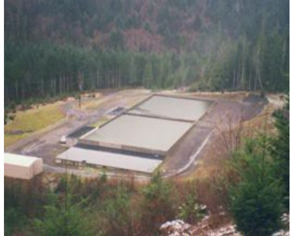
Photo of facility showing the filter basins.
