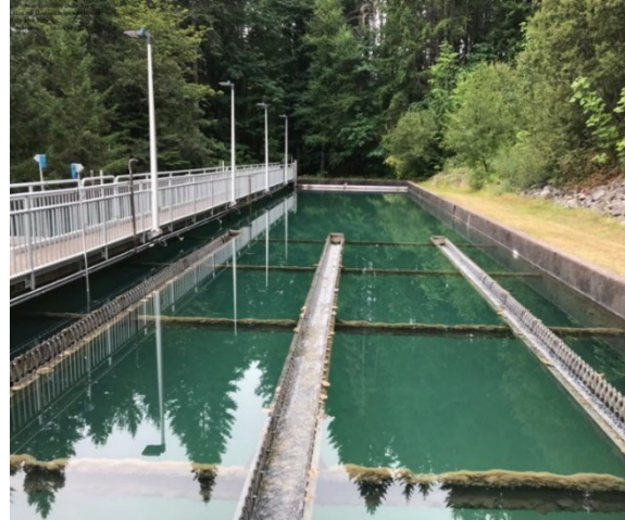
Photo of Rock Creek WTP basins.
