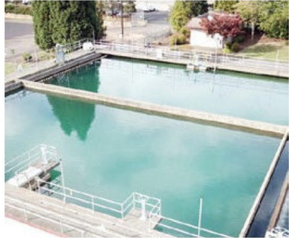
Photo of Clackamas River Water WTP with basins in foreground.
