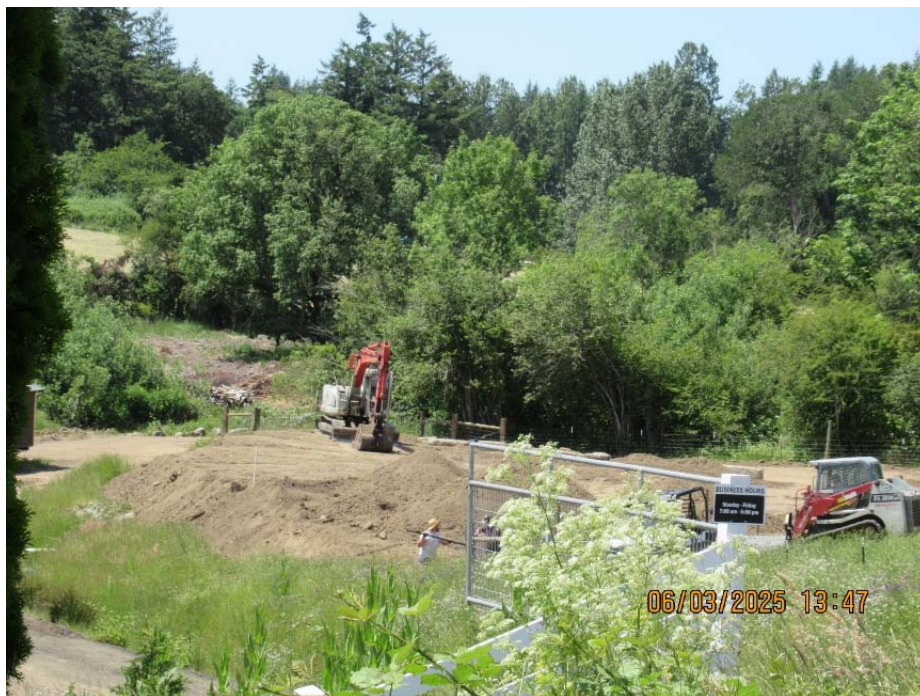
Figure 4 – Excavator moving deposited dirt on the southwest corner of property R961160130 within the SEC-s overlay
