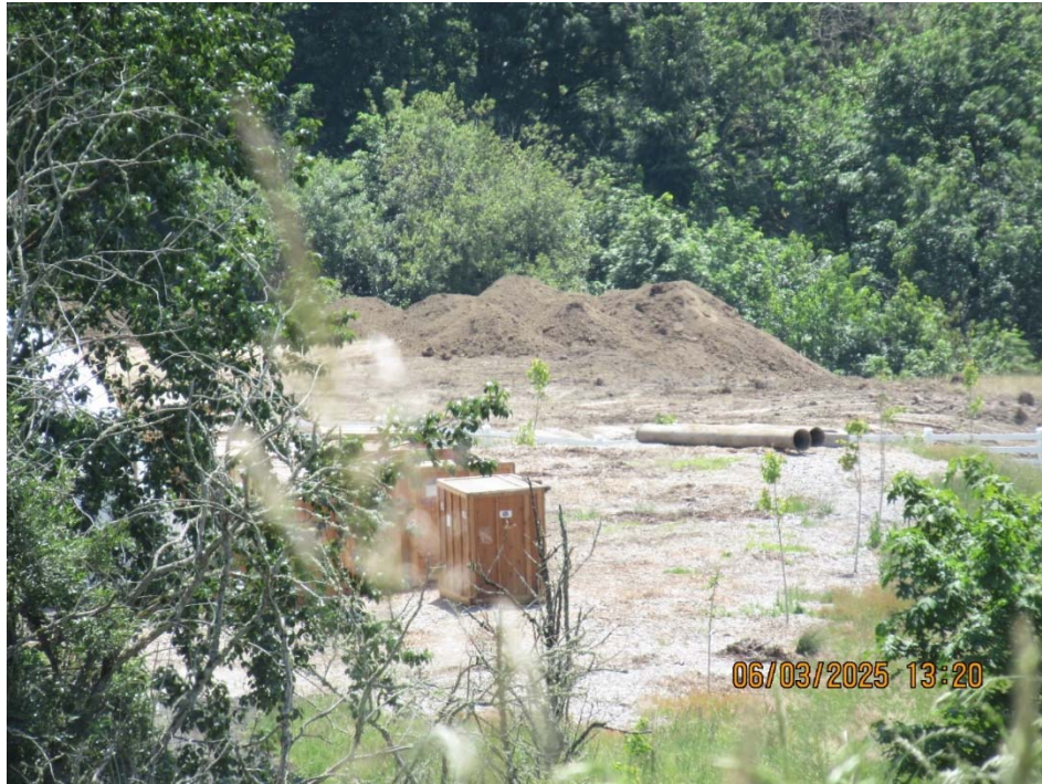
Figure 5 – Stockpiled dirt with no erosion control measures in place, located on the northern side of property R961160130
