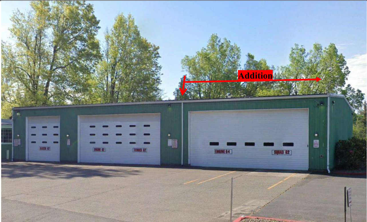
Figure 4: Front (north) elevation of Corbett Fire Station. Detail of east addition. View 166°. Photo taken on 05/12/2025.
