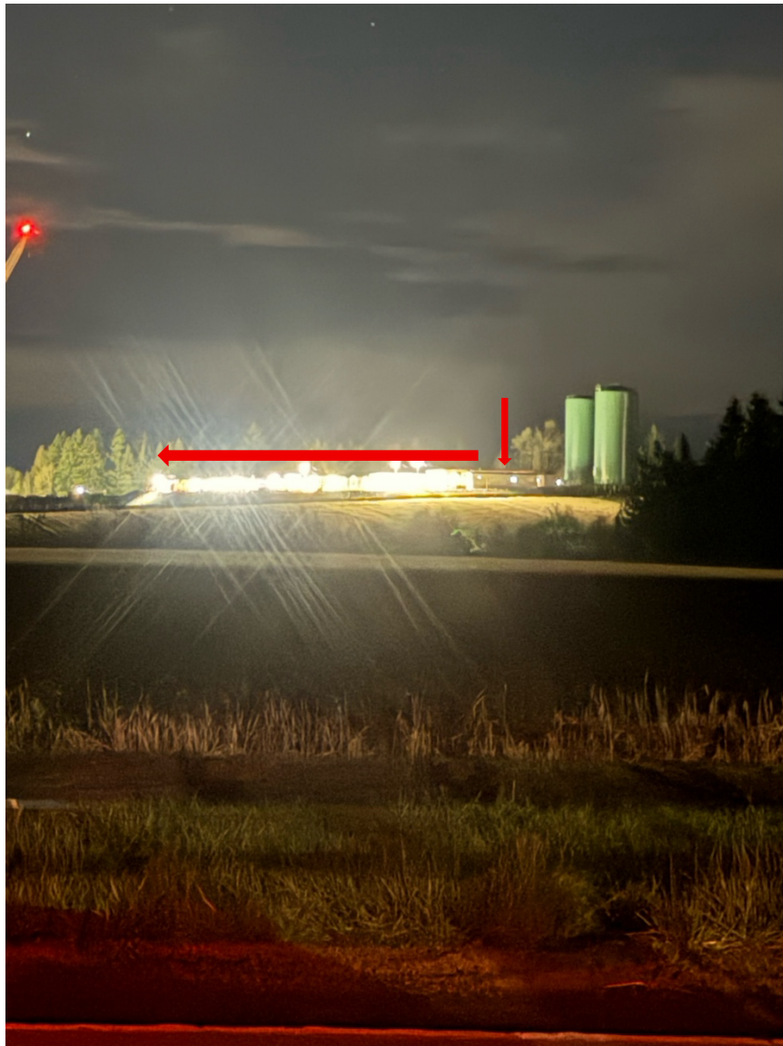
Figure 2. Photograph from SE Bluff Rd looking north, taken at approximately 7:37 p.m on March 7, 2026. Red arrows show the extent of the construction trailers at the filtration site directly west of the Pleasant Home Water District water towers.
