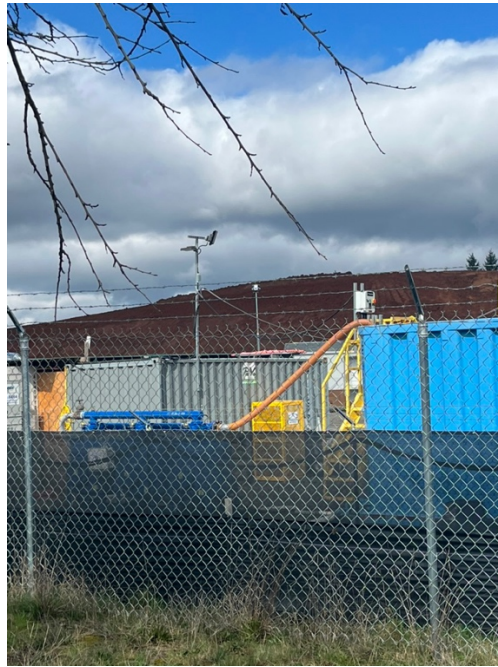
Figure 3. Light positioned in a non-downward fashion near the raw water portal on the Bull Run Filtration site immediately adjacent to residential property (photo take March 7, 2026)
