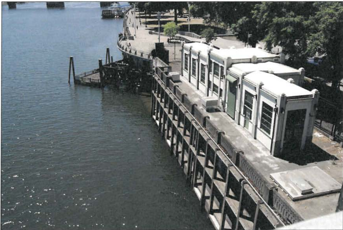
A view of the Portland Harbor Wall and the Ankeny Pumping Station taken from the Burnside Bridge; the view is towards the southwest. Note the original concrete rail panels adjacent to the pumping station.
