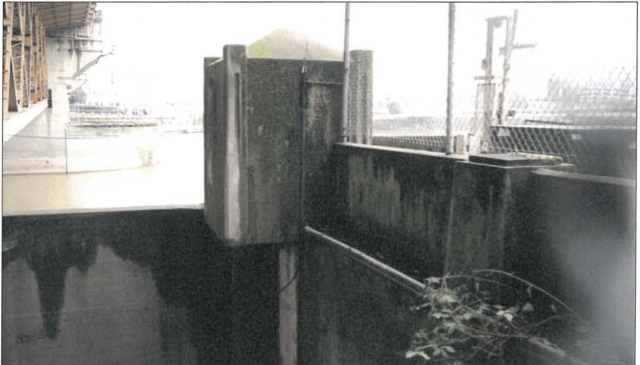
View: A small concrete structure built on the Harbor Wall south of Burnside Bridge's Pier 1, view to east.
