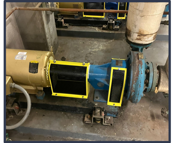
Water Pump with New Safety Guards
