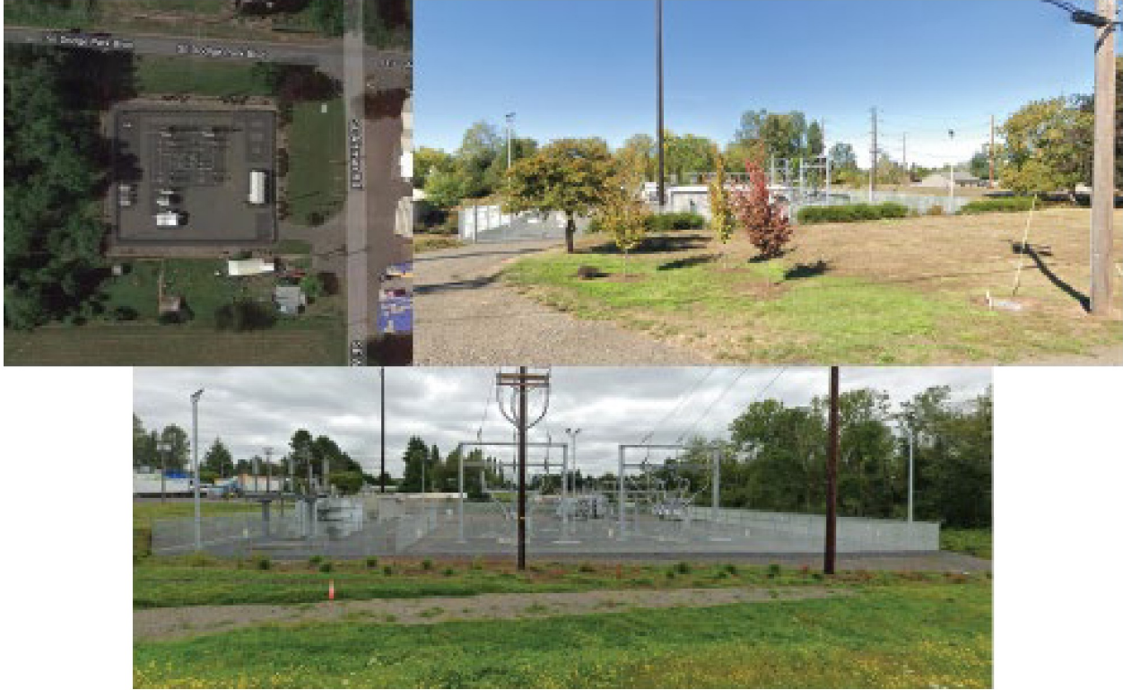
Figure 18. Electrical Substation (SW Intersection of Altman Road and Dodge Park Boulevard #12)
