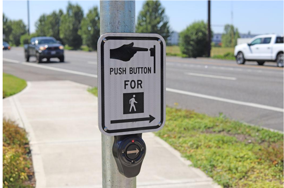
Photo of a pedestrian push button at a traffic signal
