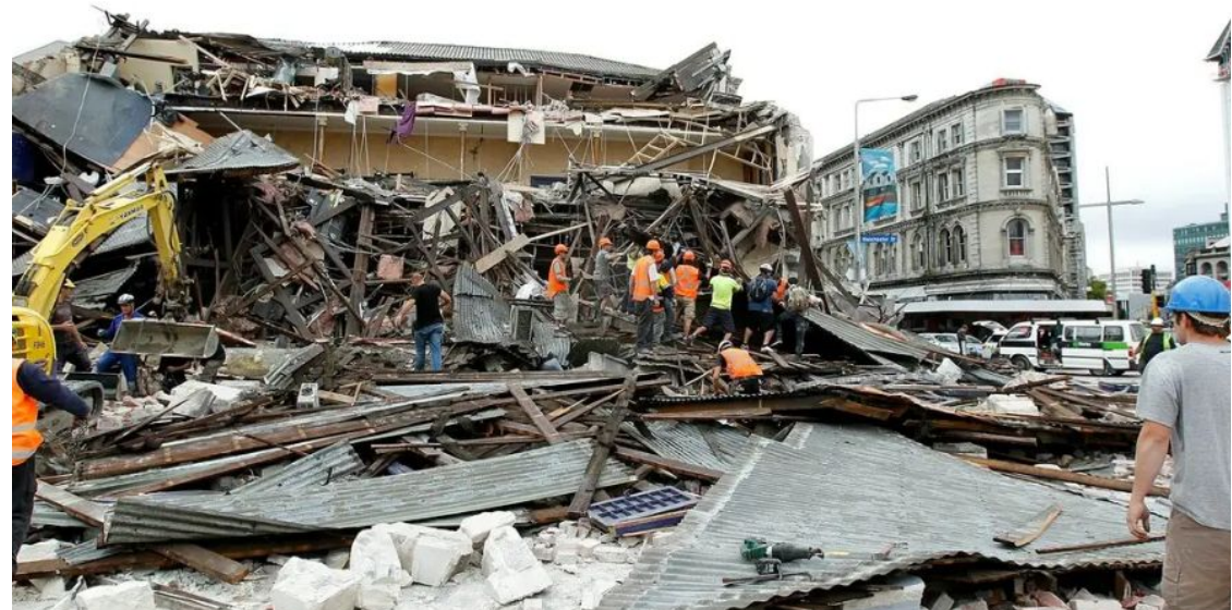
NYTimes: Damage from 2011 earthquake in Christchurch, NZ
