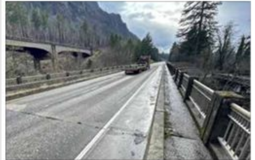
Rutting and wear on the Moffett Creek Bridge.
