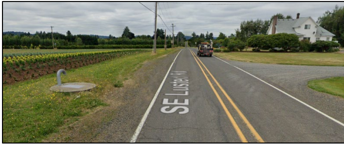
Figure 9. Example of existing air vent and access vault (left) within the SE Lusted Road right-of-way
