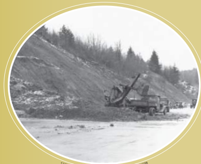
Workers remove slide debris from SW Barbur Blvd. circa 1937.
