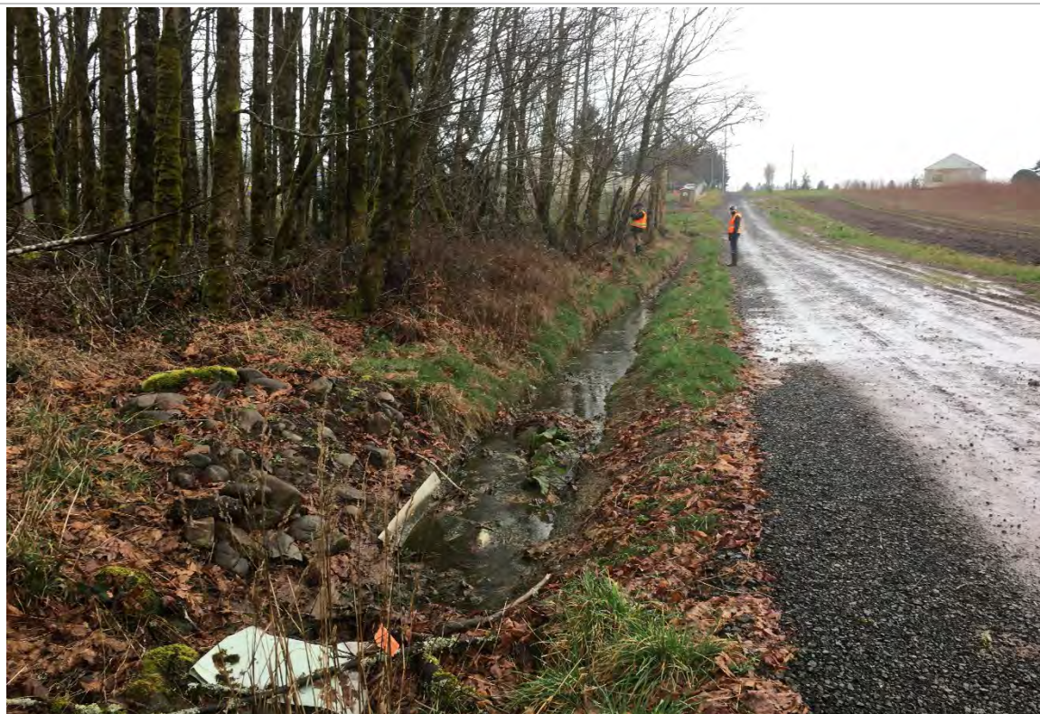
Photopoint 15: Roadside ditch/Water 4; Figure 5d. Low end of farm access road ditch during rainstorm. Plot 14 taken above ditch at edge of tree grove. Ditch inlet obscured by debris.
